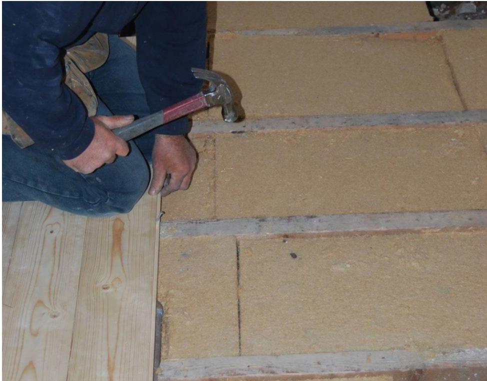
New floorboards being re-laid after wood-fibre board insulation was fitted between the joists on the ground floor of the Lodge.
